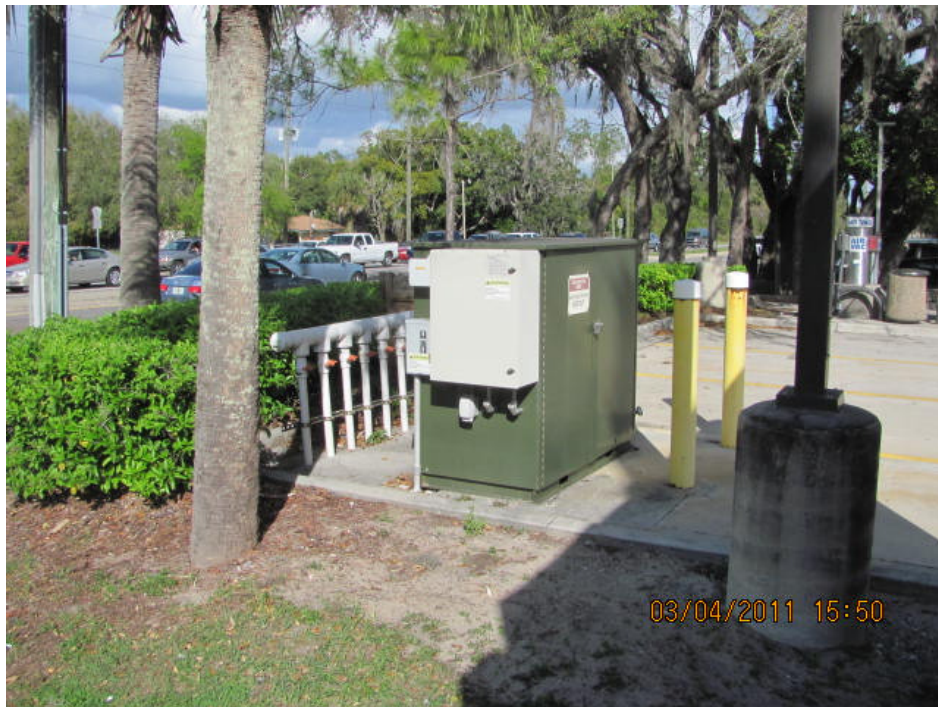
Photograph 16: Remediation system equipment at the 7-Eleven gasoline station.
